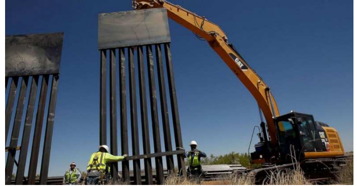
Construction workers place a panel of new bollard wall with the help of heavy machinery in Santa Teresa, New Mexico, as seen from the Mexican side of the border in San Jeronimo, on the outskirts of Ciudad Juarez, Mexico.
