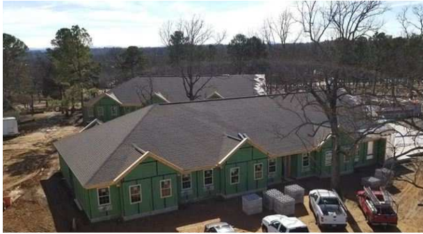
View of the new monastery being built at St. Scholastica in Fort Smith, Arkansas
