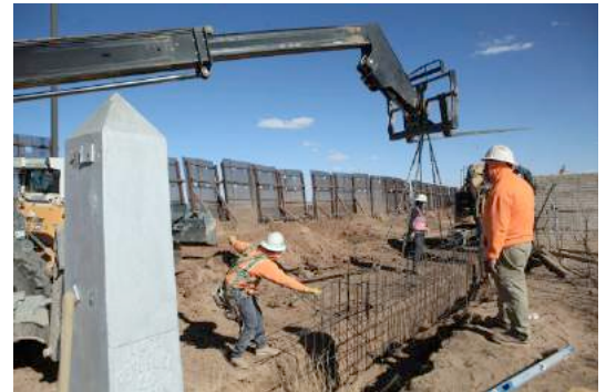
Ultimate Concrete workers constructing part of President Trump's border wall this month in Puerto Palomas, Mexico. Photo Credit: Luis Torres/EPA, via Shutterstock
